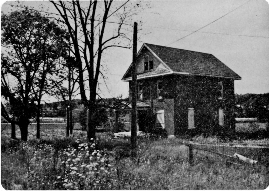
24 Below Lock No. 22, Nassau Mills, August 1978. Abandoned dwelling house formerly occupied by the Bridgekeeper and Damkeeper at Nassau below the lock station. House was used at least in 1930. 1
